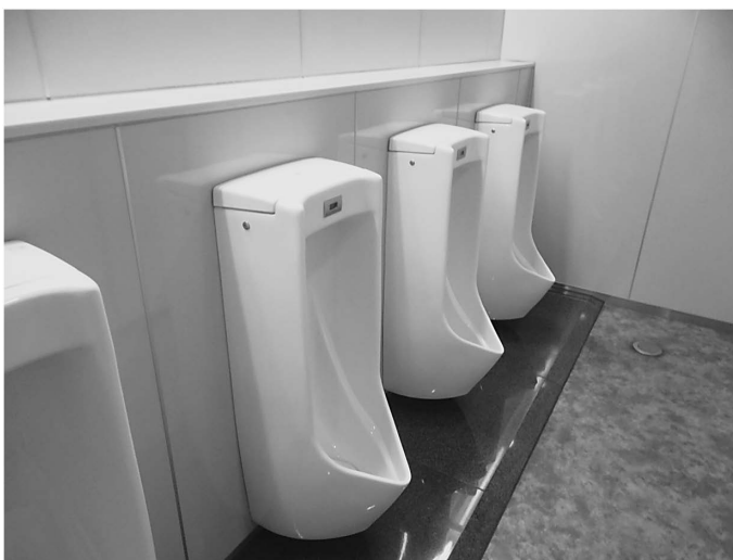
Fig. 1. Gentlemen's water closet of a variety shop in Osaka.
